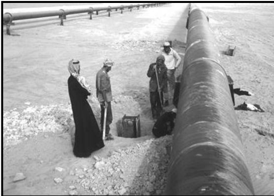
A maintenance crew attends to an oil pipeline in the Persian Gulf.
