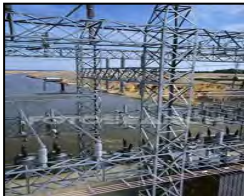
Hydro-electric power station
