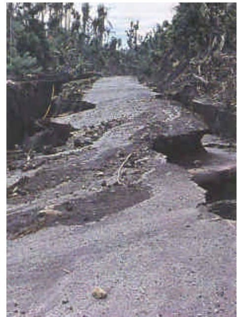
Figure 7: Rabaul road washout. Source: Lauer (1995)
