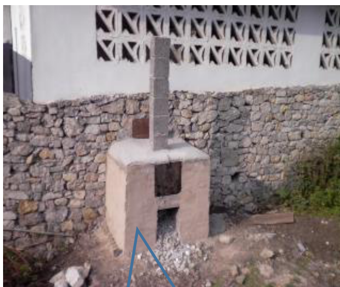
Small incinerator (Fire Box), outside of girl's toilet
