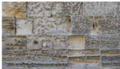
A rock wall is damaged by acid rain.
